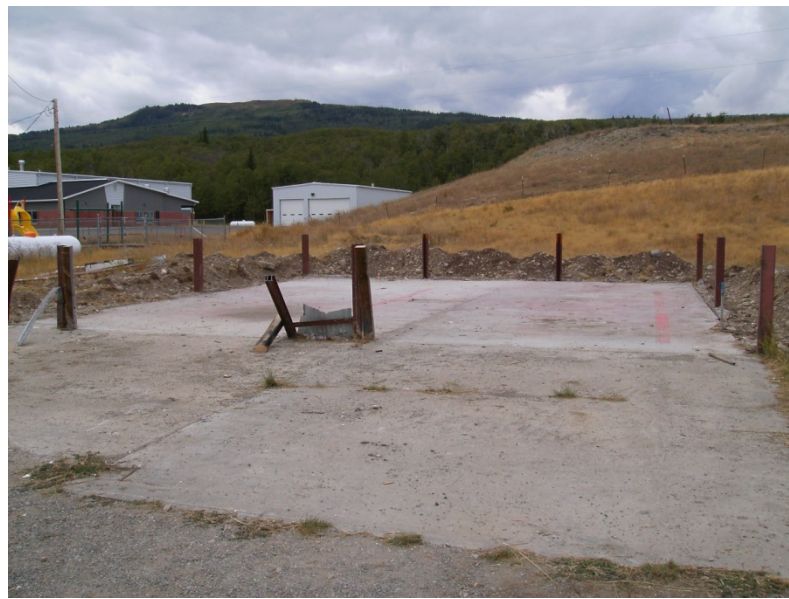
The old station 2 has been demolished and is now just an empty slab. Construction on the new station will begin soon.
